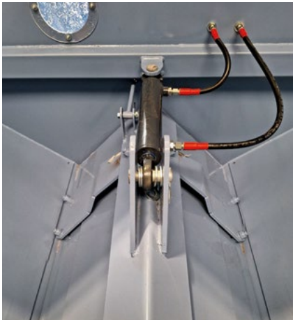
A SLIDE GATE THAT OPENS HYDRAULICALLY. IT FEEDS GRAIN INTO AN AUGER.
